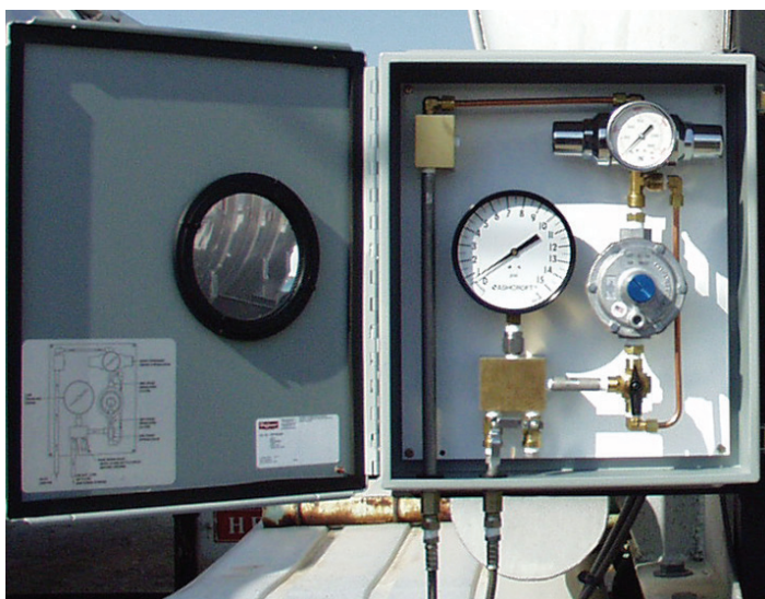
Supply and tank pressure gauges on the Mini Inert Air System are easily viewed through a large viewing port on the cabinet door.
