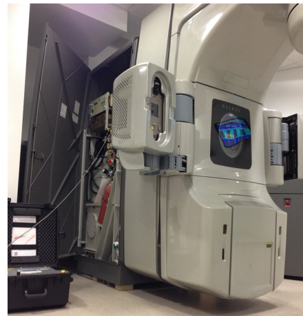
The B160R11 service unit is adapted to the requirements of small gas compartments. The photo shows the device during service works on an irradiation unit.
